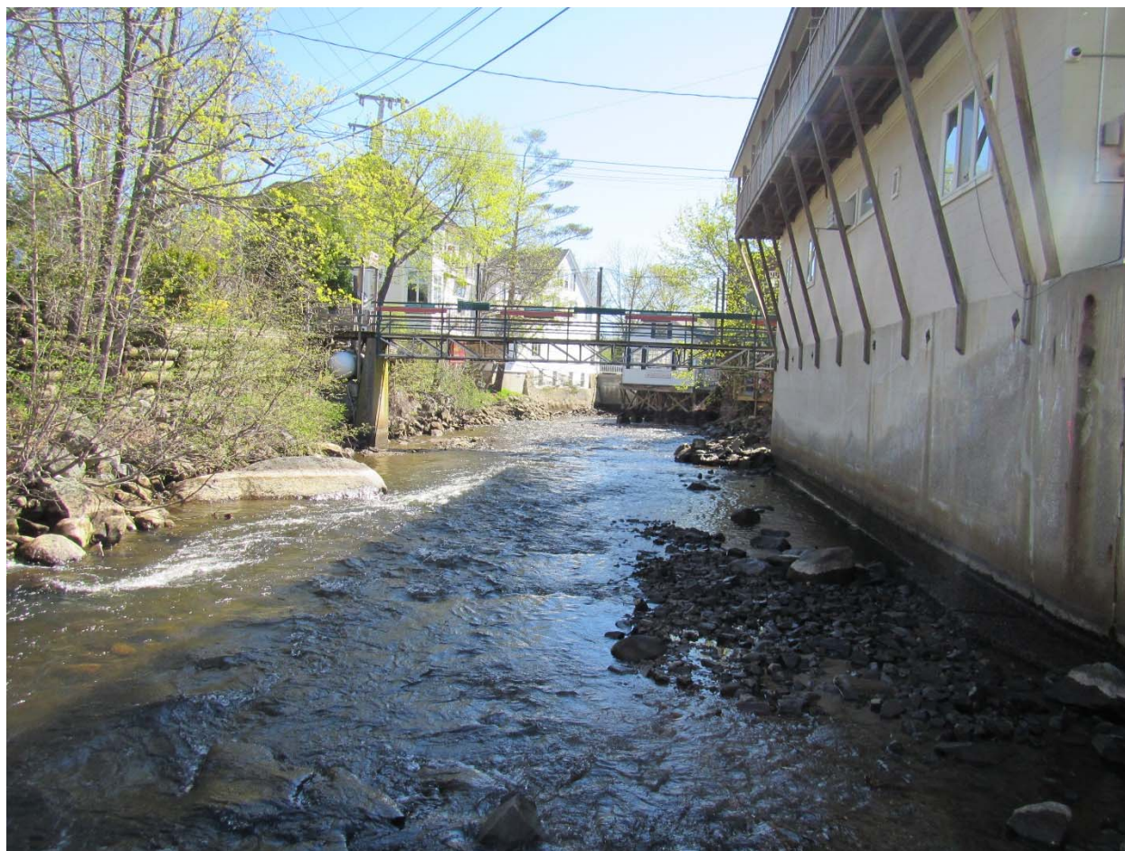
Figure 22. View of upper impoundment looking downstream from Brewster building in drawn down condition, May 8, 2018. Stain lines on large boulder at left, and concrete wall at right indicate normal pool elevation. The ground to the left of the channel is comprised of urban fill.
