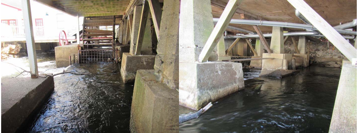
Figure 28. Looking downstream beneath Brewster building, May 8, 2018. Relict water wheels and weirs between pier footings visible in images.
