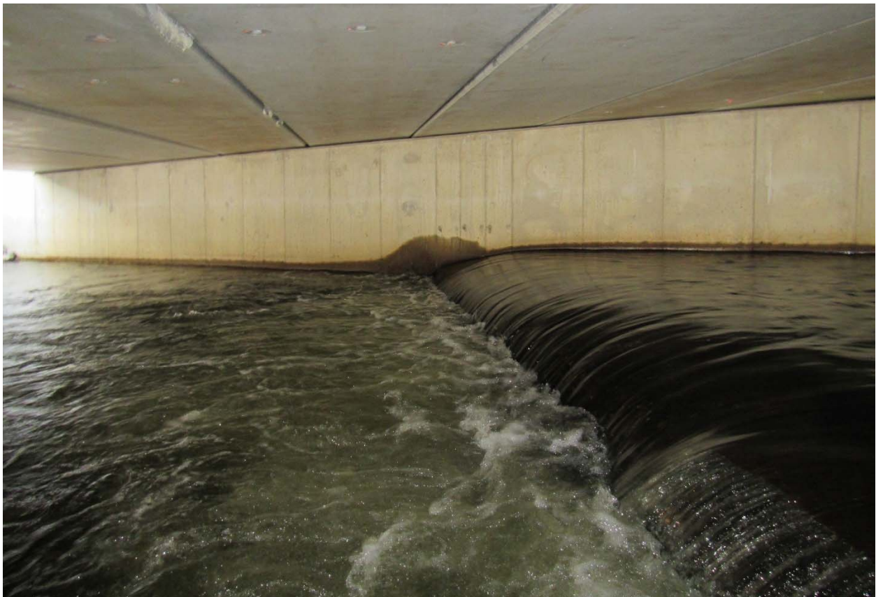
Figure 29. View across channel beneath Washington Street bridge, May 8, 2018. Concrete sewer line encasement creates hydraulic drop of approximately 9 inches.
