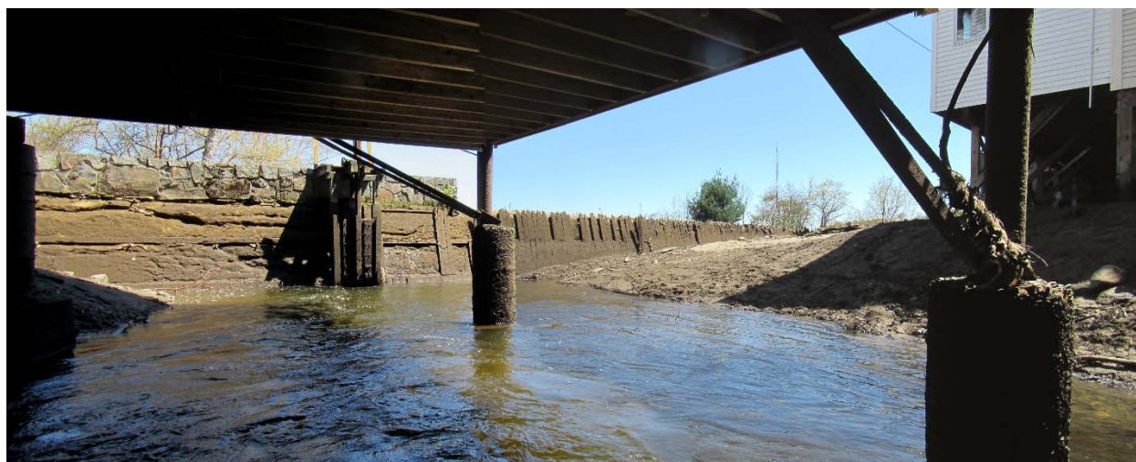
Figure 21. View of lower impoundment in drawn down condition, May 8, 2018. Non-overflow portion of dam and headgate at left half of image, spillway at right half of image. Normal pool elevation at spillway crest.
